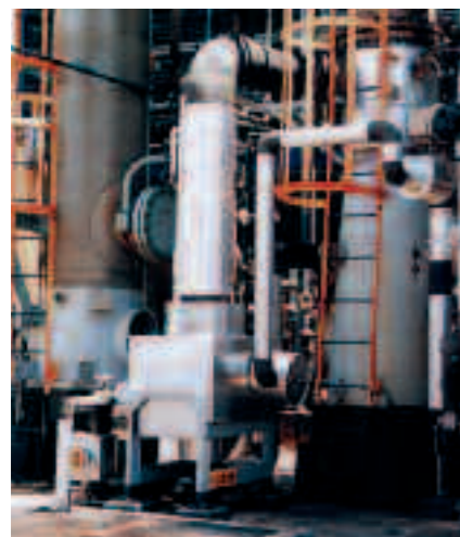
Compabloc installed as stripping column reboiler at an ethyl-acetate plant in Rhodia, Brazil
