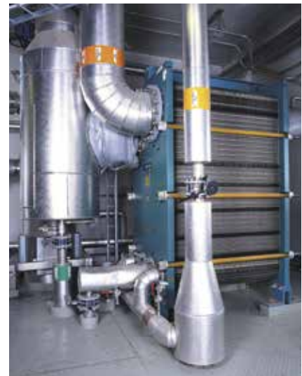
Ethanol condenser at The Absolut Company in Sweden. All the columns at The Absolut Company's Åhus distillery use Alfa Laval reboilers and condensers. The Alfa Laval units were chosen because of their compactness compared to corresponding shell-and-tube solutions.
